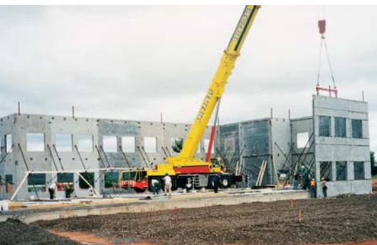
LEFT: Tilt-up concrete panel erection at Northeast Kings Education Centre, Canning, NS
