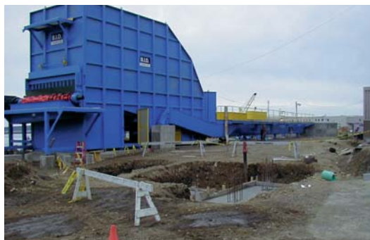
Bowater’s new truck dumper is a major component of their $4-million chip conversion project.
